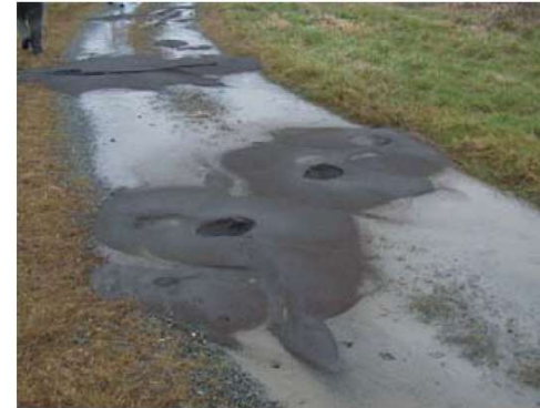
Sand boils , Nisqually wildlife refuge
